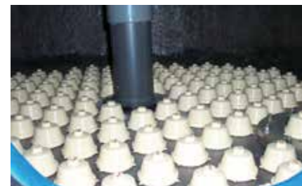
Nozzle Plate under drain system
