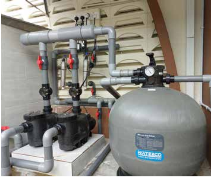
Waterco filter system installed at Masjid Muhammadi Kota Bharu, which consists of a Micron Top Mount Fibreglass Filter S700, two Hydrostorm 100 pumps, an insect trap and a UV steriliser.
