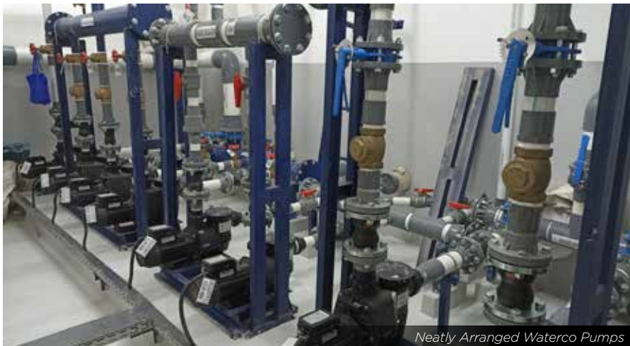
Neatly Arranged Waterco Pumps
